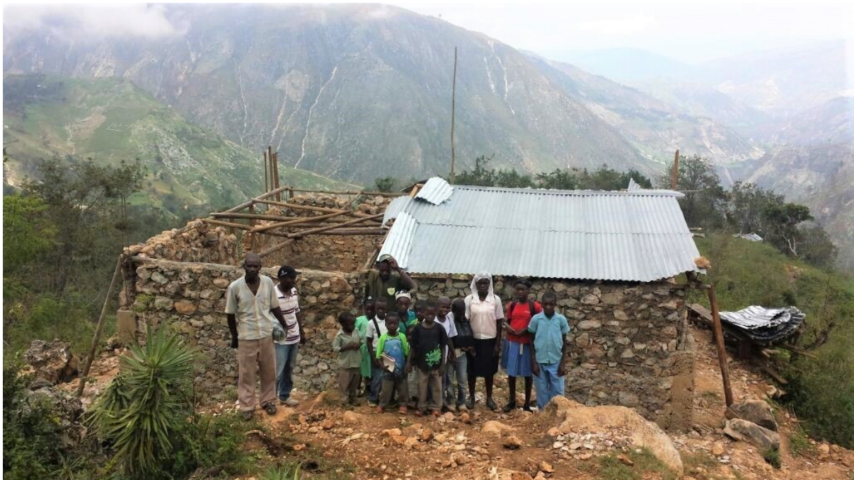
Picture 1: A family standing in front of their partly reconstructed house after hurricane Matthew. Haiti 2016. Helvetas Swiss Intercooperation
