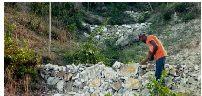
Installation of dry barriers to stabilize the bed of ravines (HELVETAS Swiss Intercooperation)
